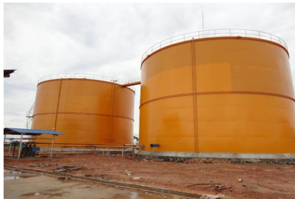
CPKO storage tanks
