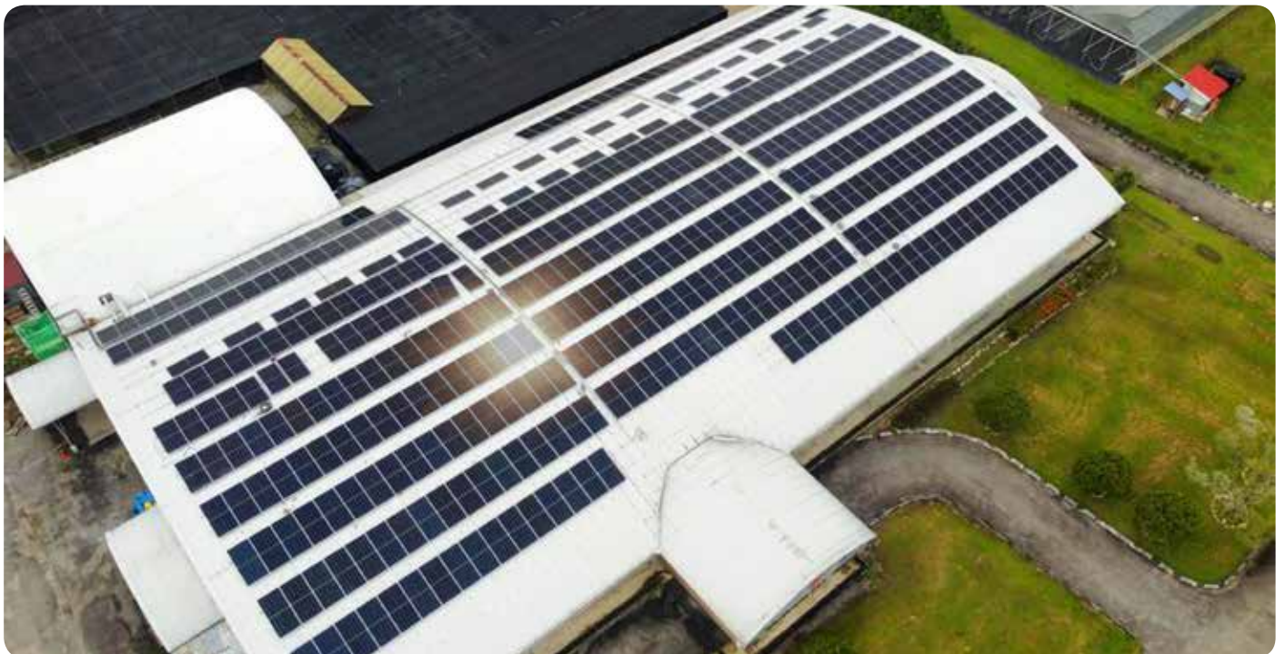
Rooftop solar panels at our R&D centre in Banting, Selangor, Malaysia.
