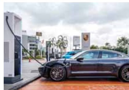
Porsche Centre in Malaysia became the first to offer 175kW High Performance Charging infrastructure as part of a its commitment to drive the future of electric mobility in the region.
