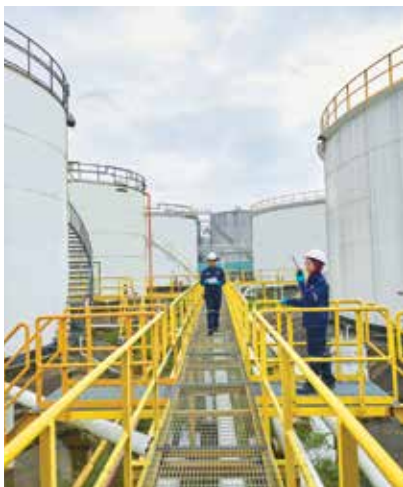
Driven by operational excellence, our plant and terminals continue to deliver flawless operations to ensure seamless terminal throughput and delivery
