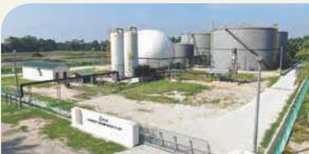
Biogas Capture Plant
