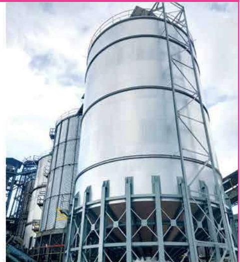
New 1,000 mt Kernel Bulk Silo.
