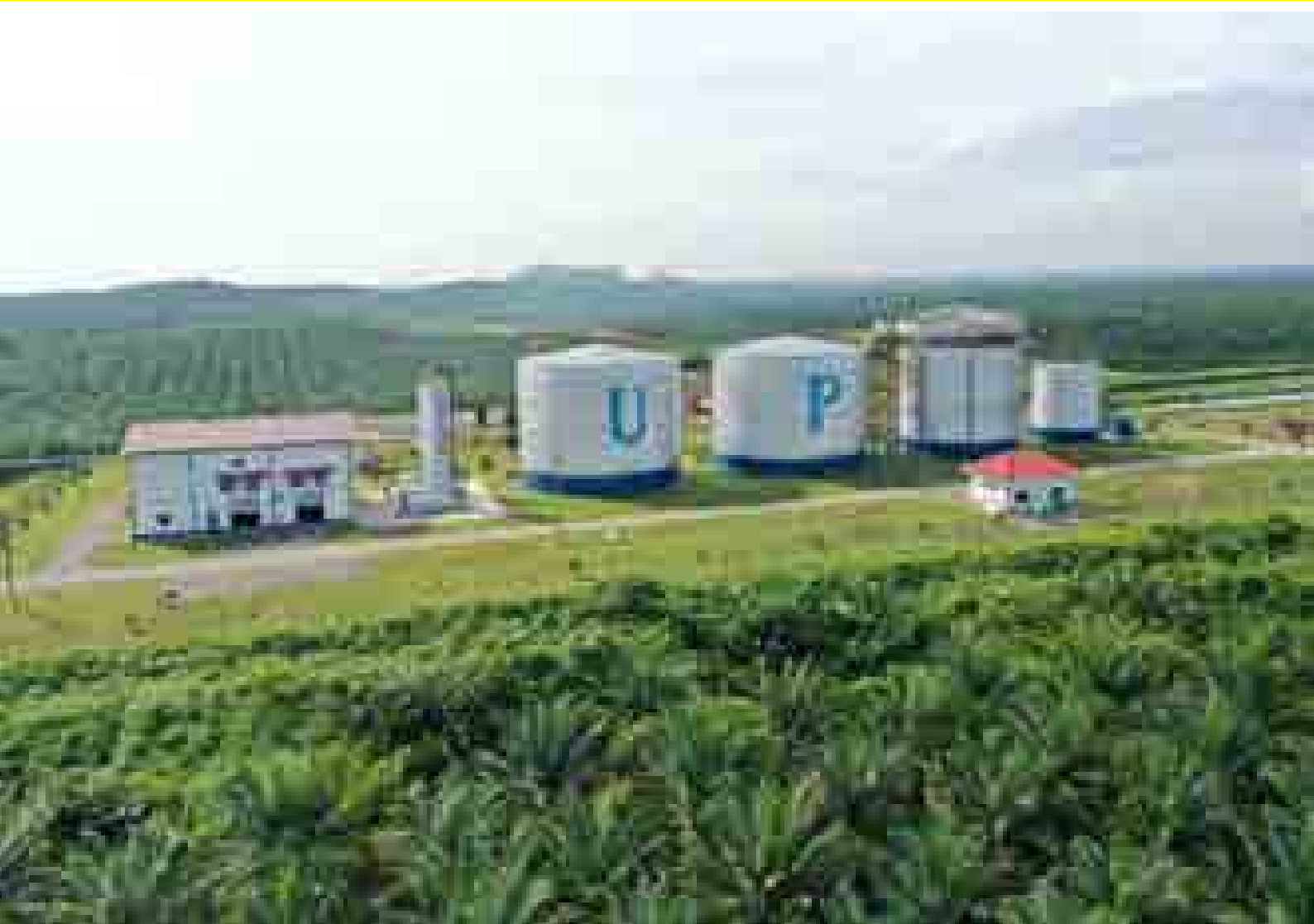
In line with our commitment of reducing GHG emission, all UP's Palm Oil mills are equipped with Biogas Plants. The above is situated at the Optimill in Ulu Bernam.
