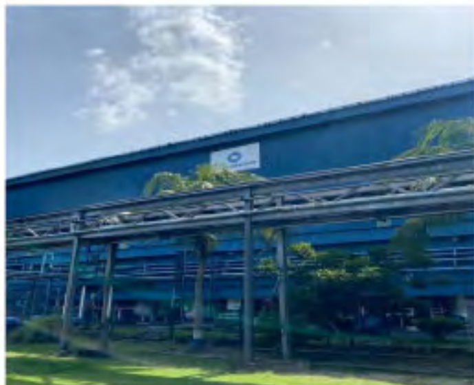
Rain gutter is installed beside the roof of the Palm Kernel Dry Fractionation Plant (“PKDF”) to collect rainwater, that flows by gravity into catchment pond.
