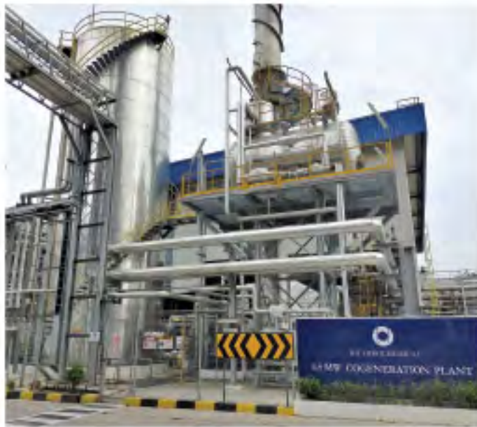
Our CoGeneration Plant in Johor
