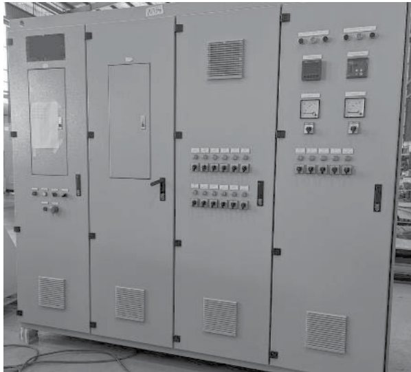
Process control panel
