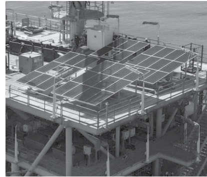
Our Ex solar PV system installed on an O&G platform
