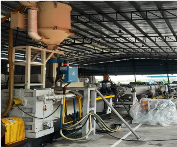
View of mixing tower of pipe extrusion line, dried raw materials (being HDPE resin and masterbatches) will be loaded
