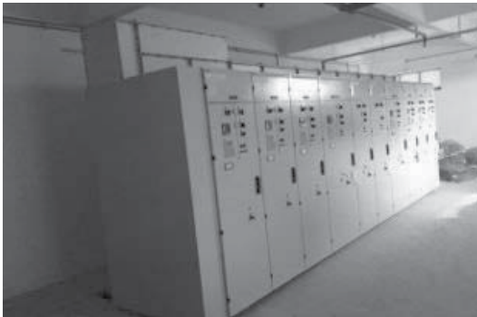
33kV medium voltage switchgear panel
