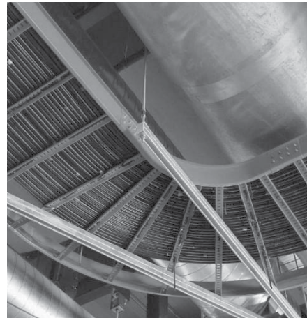
Electrical wiring system
