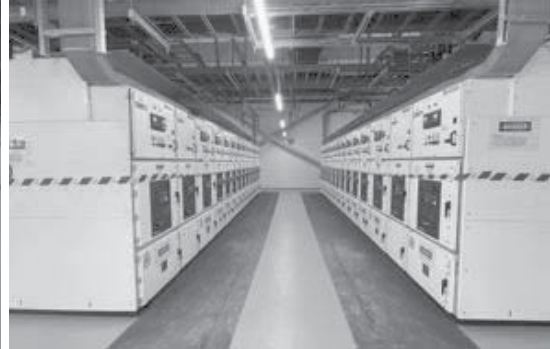
11kV medium voltage switchgear panel
