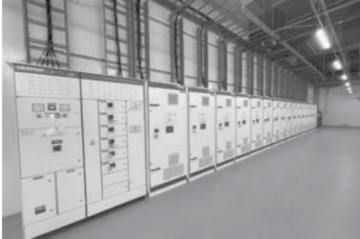
Low voltage main switchboard panel
