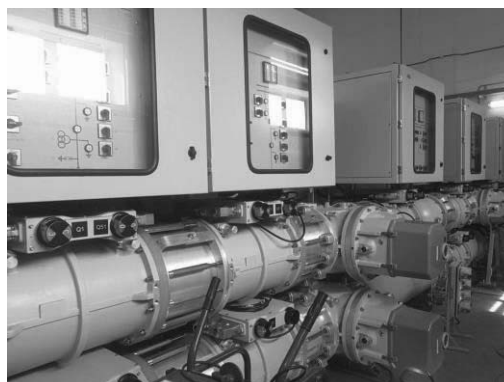
132kV gas insulated (GIS) substation for a semiconductor manufacturing plant
