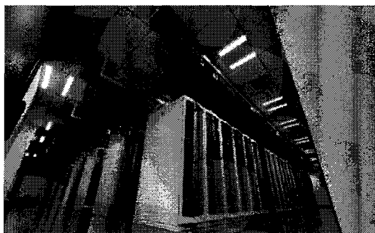
Final positioning of the server and network racks in data centre
