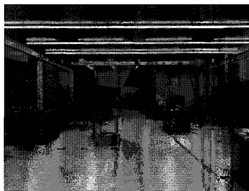
Class 1,000 ISO 6 cleanroom project for a semiconductor manufacturing facility in Batu Kawan Industrial Park, Pulau Pinang
