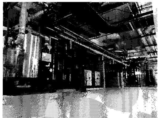
Plantroom project for a semiconductor manufacturing facility in Bayan Lepas Free Industrial Zone Phase 4, Pulau Pinang
