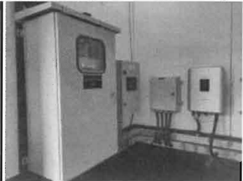
Our energy management system installed as part of a solar PV facility
