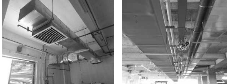
Fire sprinkler systems
