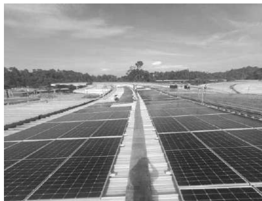
Overview of a rooftop solar PV installation
