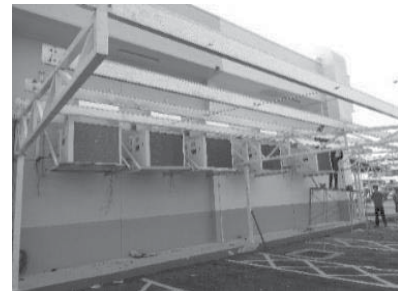
Air conditioning compressors
