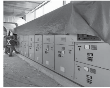
Motor control centre panels
