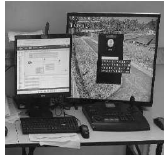
Remote security monitoring system
