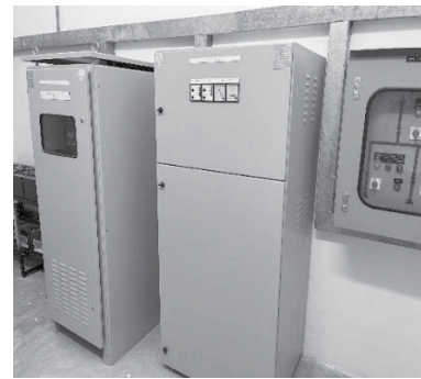
Distribution boards for energy management systems
