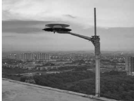
Lightning rod protection system
