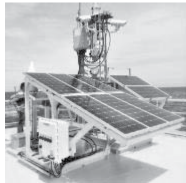
Ex navigational aids system with solar power supply
