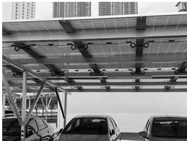
Installation works for solar PV on a car park in Shah Alam, Selangor
