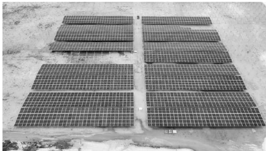
Mechanical installation works of the structure and mounting frames for the development of 50 megawatt alternating current (MWAC) solar PV facility located in Pekan, Pahang
