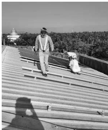
Installation works for solar PV panels on a rooftop in Kuala Langat, Selangor
