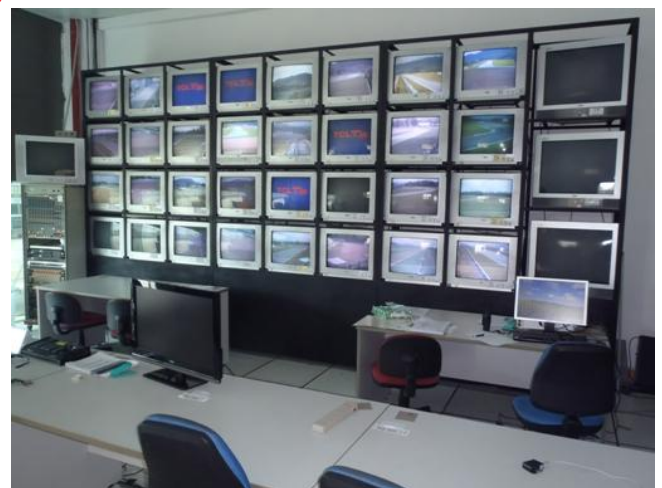
Figure 8: ZIC control room
